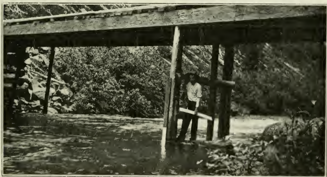
Installing metal-faced gauge at metering section on Sumallo river one mile from mouth.
